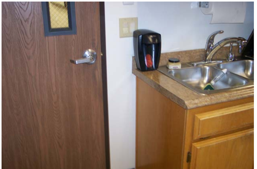
B1. Employee Lounge Door Encroachment
