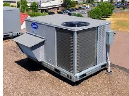
New Roof-top unit
