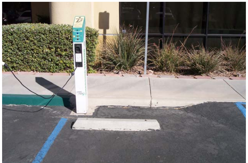
F1. South EV Charging Station Encroachment
